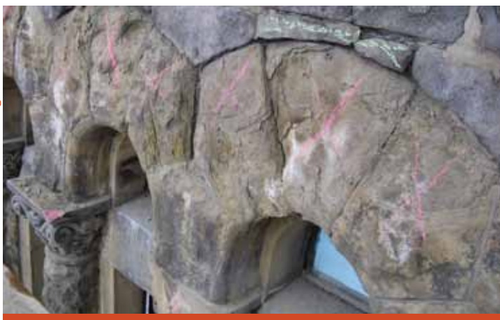
Stonework in the bell tower was marked for replacement (left). The impressive results (right) included careful cleaning and repointing.
