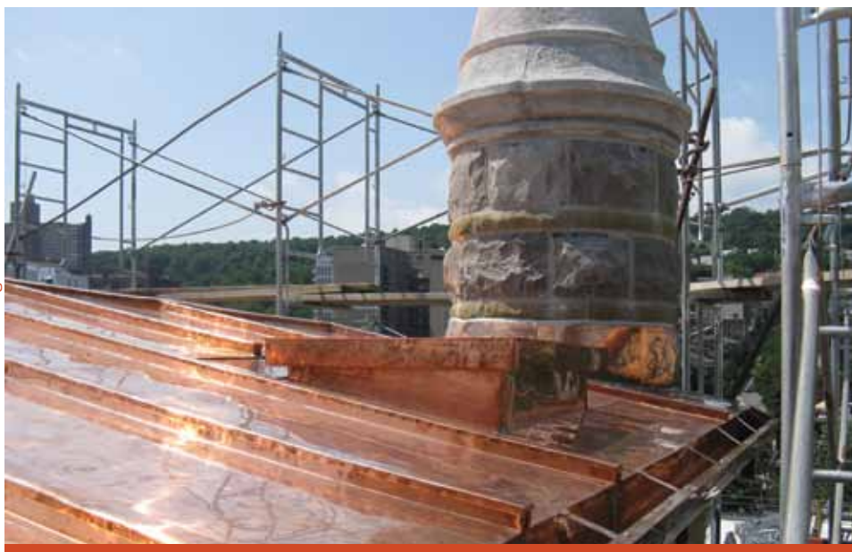
A new copper roof was installed on the bell tower. To ensure better control of water runoff and reduce erosion, new flashings were mounted.
