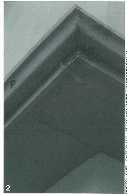
Soffit with wood deterioration.
