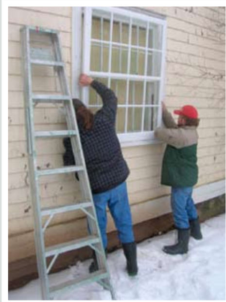
New storm window being fitted to the exterior of Runciman House, Annapolis Royal, NS, owned by the Heritage Canada Foundation.
