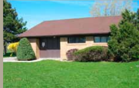
Substation House Scarborough
