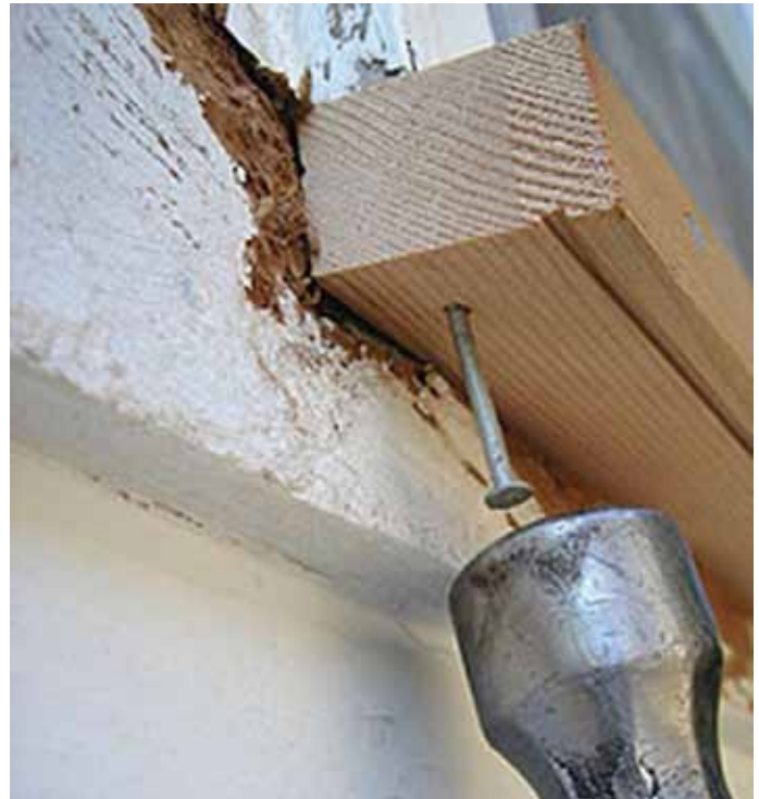
The "drip groove" under the windowsill prevents water from reaching the wall.
