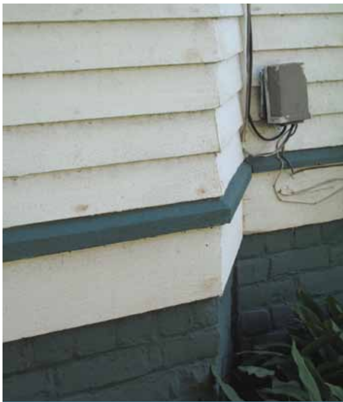
Example of a continuous “water shelf” that slopes away from the shingled siding.
