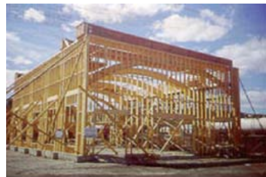
The shell, to which the hall was attached, is seen under construction.
