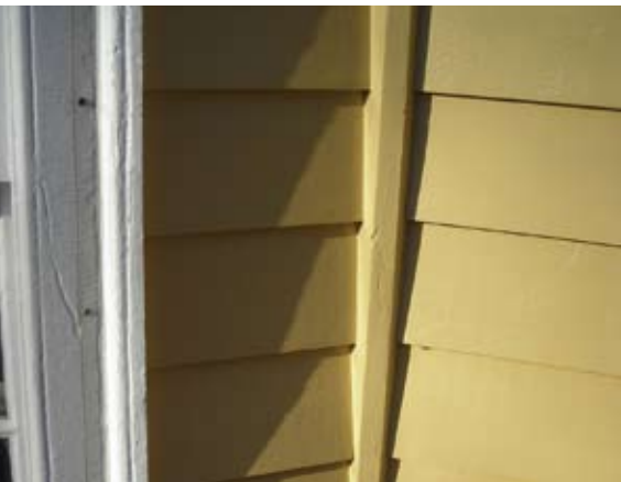
The short wood sections beside the projecting bays at the front of the house were replaced with new material.
