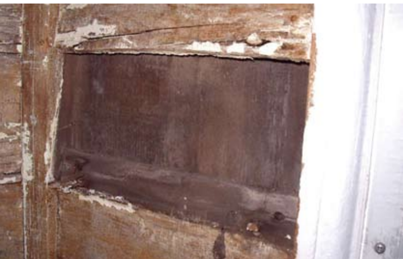
Examples of buckled and cracked siding, and popped nails.
