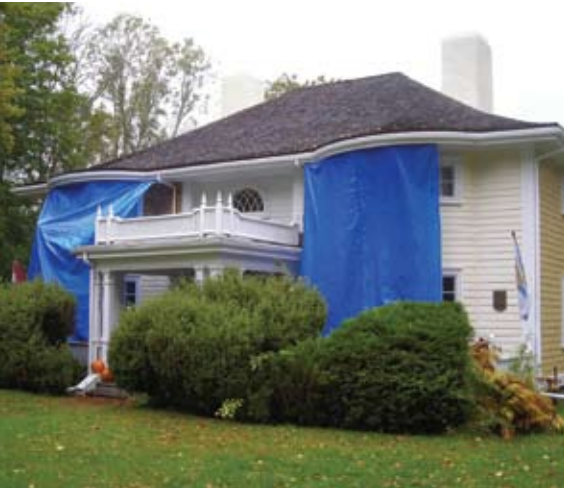
The front of the house was draped for protection prior to starting work.
